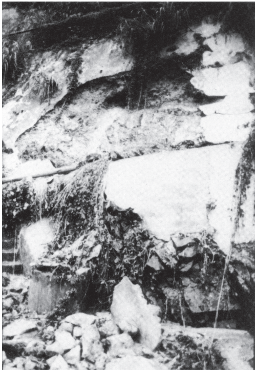
Figure 1. Pipe in Hong Kong cut slope at the boundary between colluvium and weathered tuff, which caused the hard surface protection to be blown off
